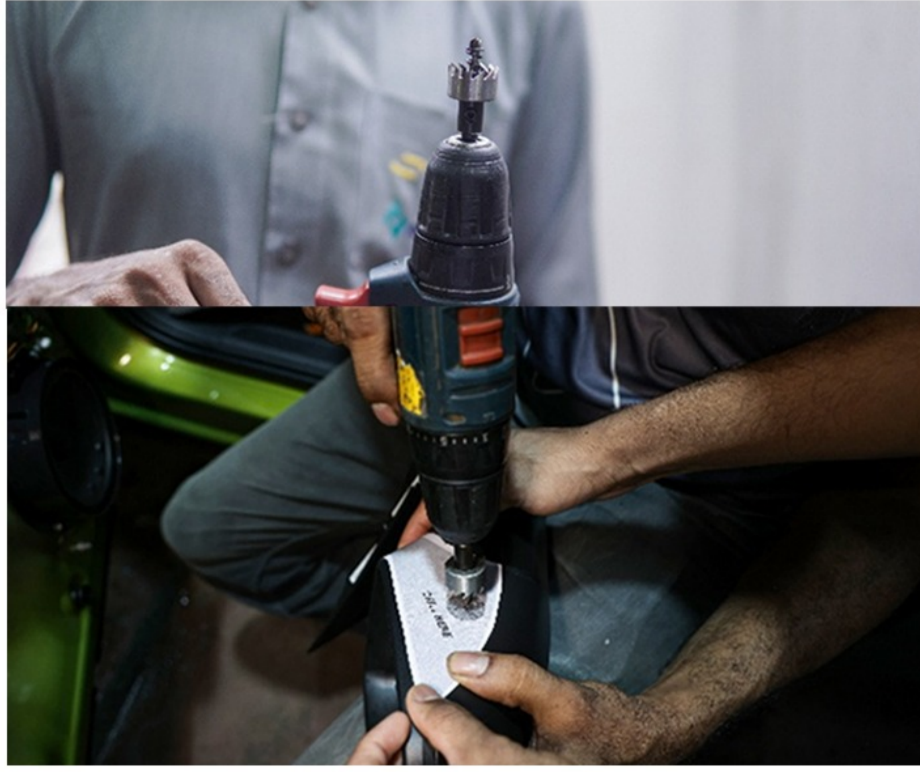
Step 33 :- Drill the hole using hole saw (part 13) as per markings given on the template
